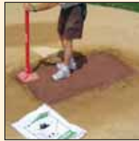
Apply a thin layer of Professional Mound Clay (match color to blocks) moisten, tamp.
