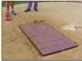
Install MOUNDMASTER Blocks, tamp, water and allow to soak in for 20 minutes.
